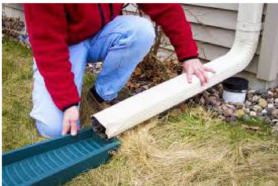
Direct runoff to unsealed ground.
